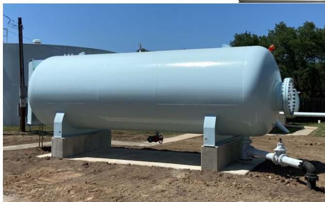
Plant 2 Hydropneumatic Tank
